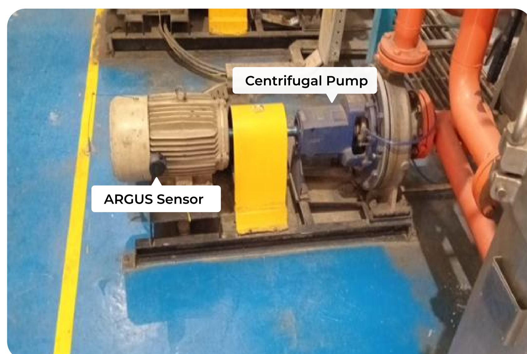
Figure 1: Centrifugal pump under monitoring
